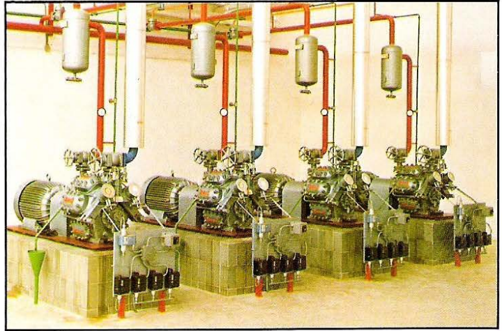
Fish industry in Spain with HC 8-75 compressors.
