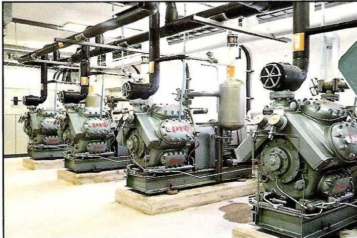
Skating rink plant at Skutskär, Sweden, with HC 8-125.
