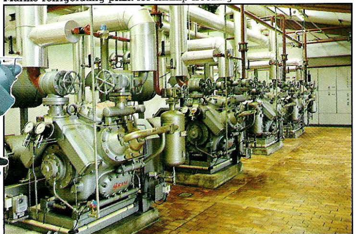
Fish freezing plant with HCT-125.
