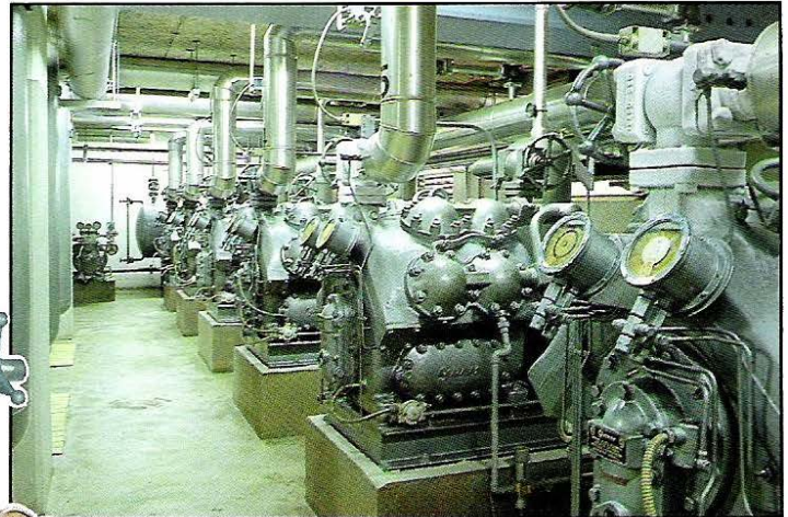
HC-800 compressors in a Danish slaughterhouse.
